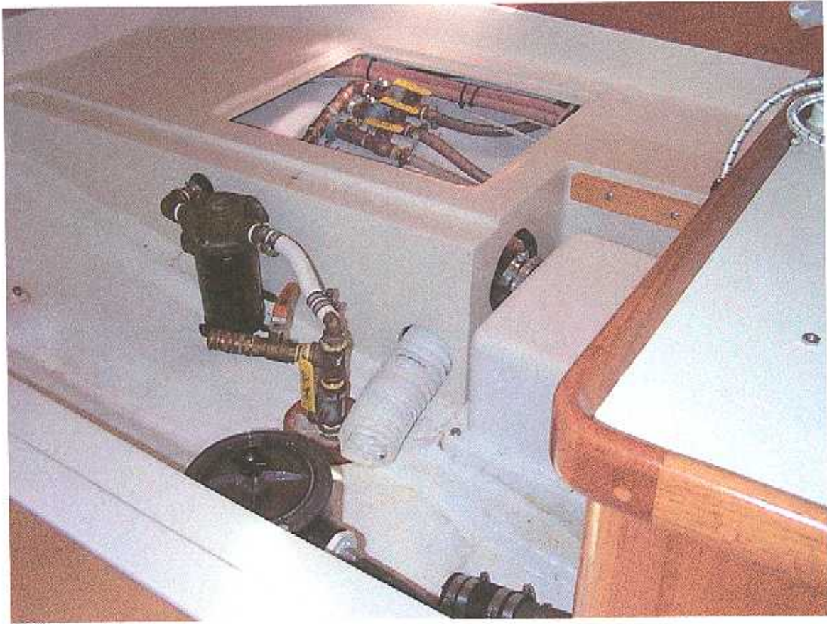
Fig 2.3 Accessory seawater seacock and manifold – general layout – Aft cabin looking toward the port quarter.
